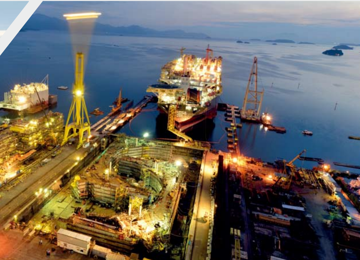
Keppel O&M has a proven track record of offering a full range of offshore and marine solutions, including the fabrication and integration of topside modules for FPSOs. This is the fabrication and integration of topside modules for the FPSO Cidade de Sao Paulo
