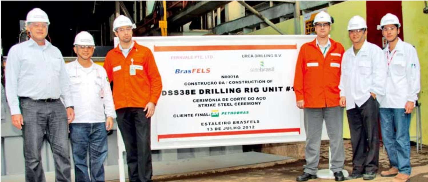
Representatives from Petrobras, Sete Brasil and Keppel FELS Brasil mark the strike steel milestone of the first of six DSS™ 38E semis on 13 July 2012 at Keppel's BrasFELS yard
